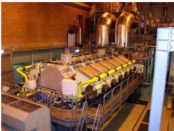
The converted 51/60DF engine at the TMG SPE co-gen plant. The newly installed gas supply lines are clearly visible in their mandatory yellow colour coding.
